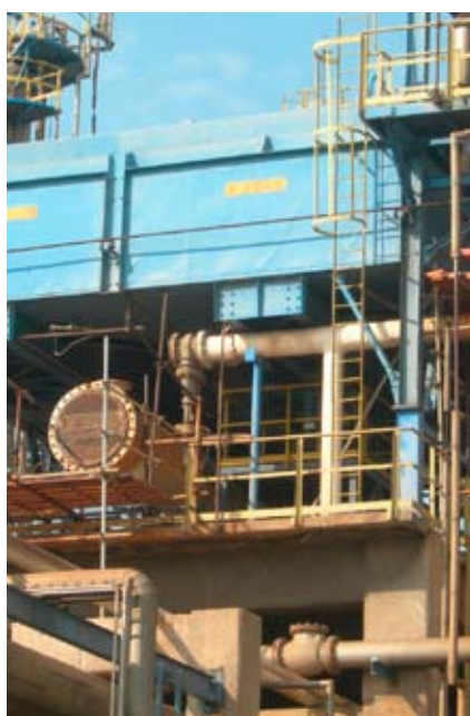
An old shell-and-tube installation
