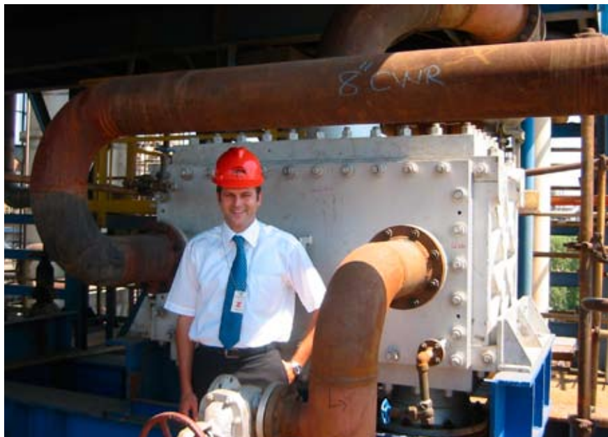
Trim condenser/subcooler for the hydrotreater unit
