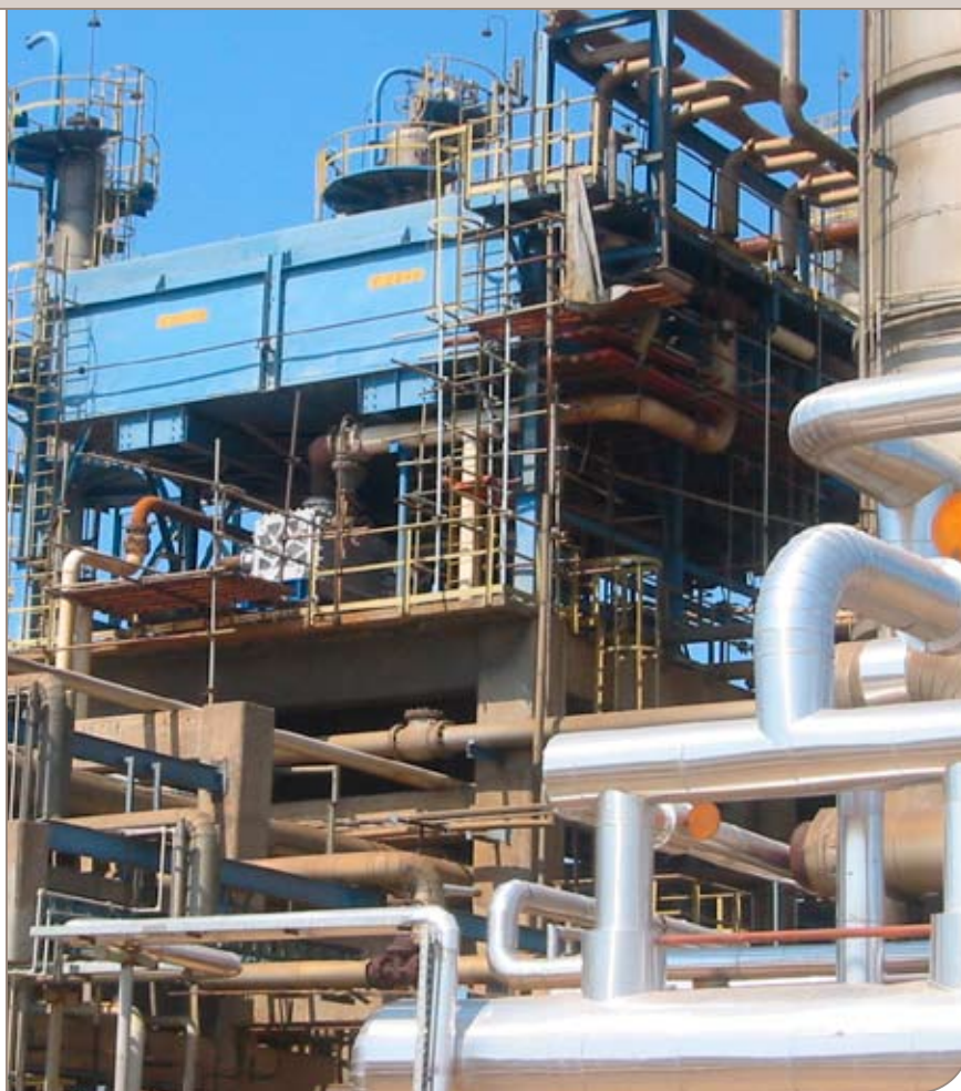
One of the two new space-saving Compabloc installations
